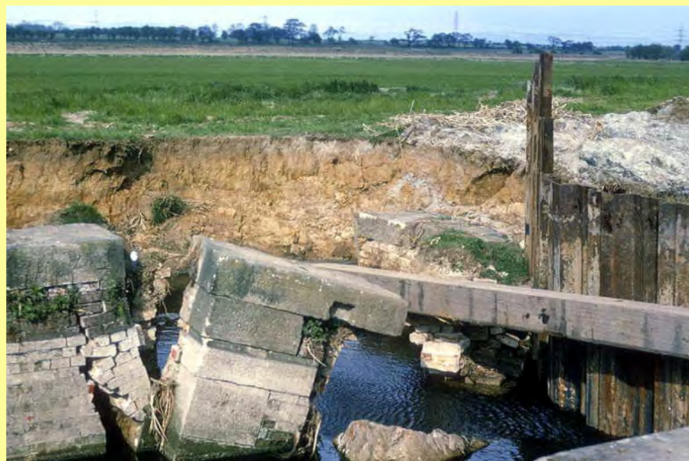
This page: There was a 'hick-up' during the restoration in 1974 when a breach occurred in the lower wing wall. This did not delay the re-opening a year later.
