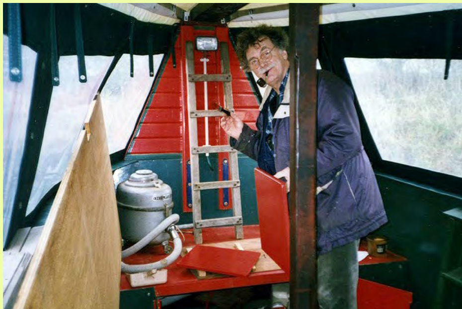
Above: A volunteer painting some of the fixtures and fittings but there was still lots of work to do before the boat was ready for the water.
