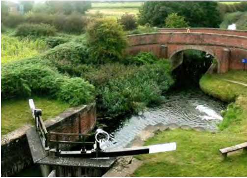
Above: The view below the lower gates at Coates Lock, taken on the 27th April 2003
