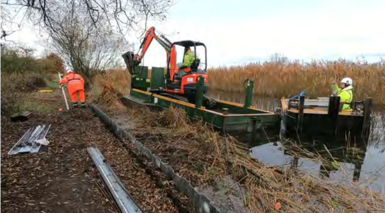
Above & Right: CRT Contractors working from the water, installing new aluminium piles above Walbut Lock on the 27th November 2023
