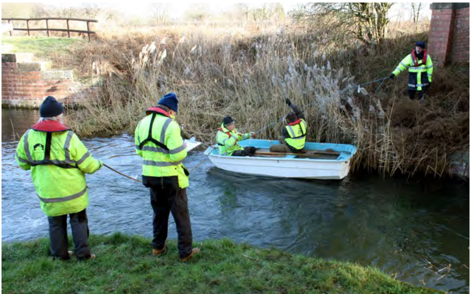
Above: Working party volunteers check the water and silt depths prior to dredging this section at Coates lock on the 31st January.
