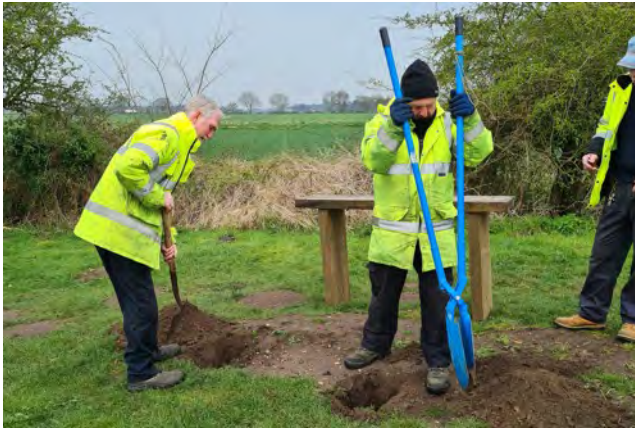
Left: Excavating the holes for the new bench at Bridge 8. 12th April 2022.
