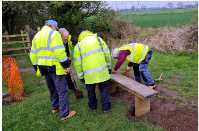
Right: The new bench is put in place. The team are checking that it is level and firm.
